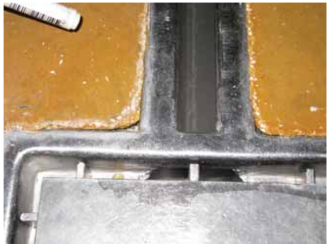
Figure 3. Sharp angles and a lack of flexible sealant where the resin floor meets the channel create crevices that can retain contaminated water.
